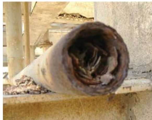
Figure 5. End View of 2" Dummy Leg from Figure 4 Shows a Heavily Corroded Internal Surface
