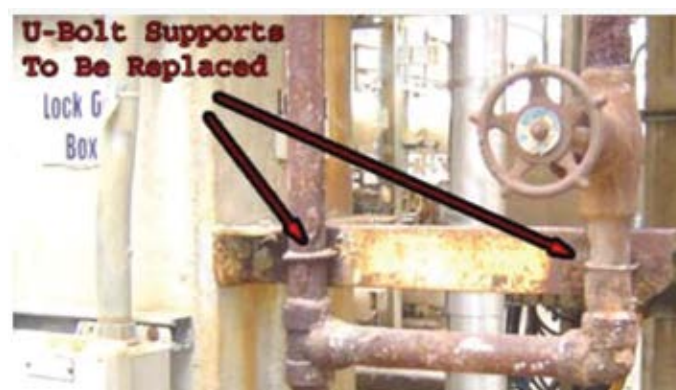
Figure 3. Severe Deterioration and CUI Visible After Insulation Removed from Piping
